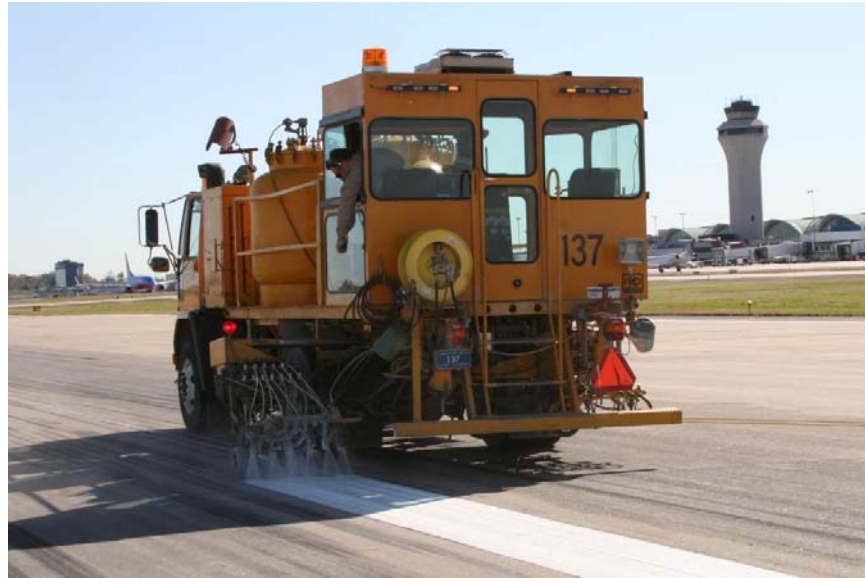
A Lambert airfield worker lays down a new centerline stripe on runway 12R-30L.
