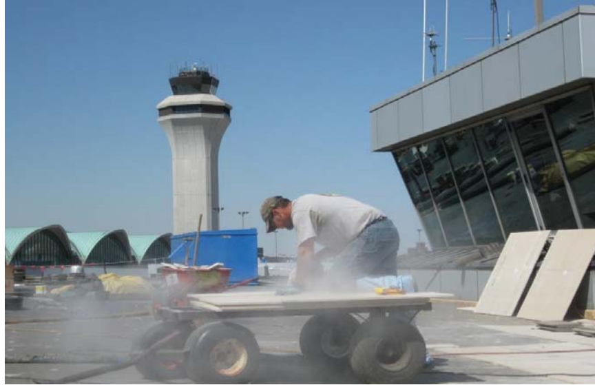
A worker cuts decking material for placement on the C Concourse roof.
