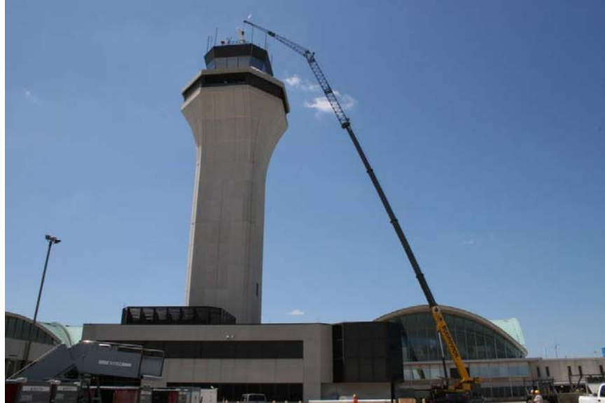
A crane skies above Lambert's Air Traffic Control Tower to deliver a new radar antenna.
