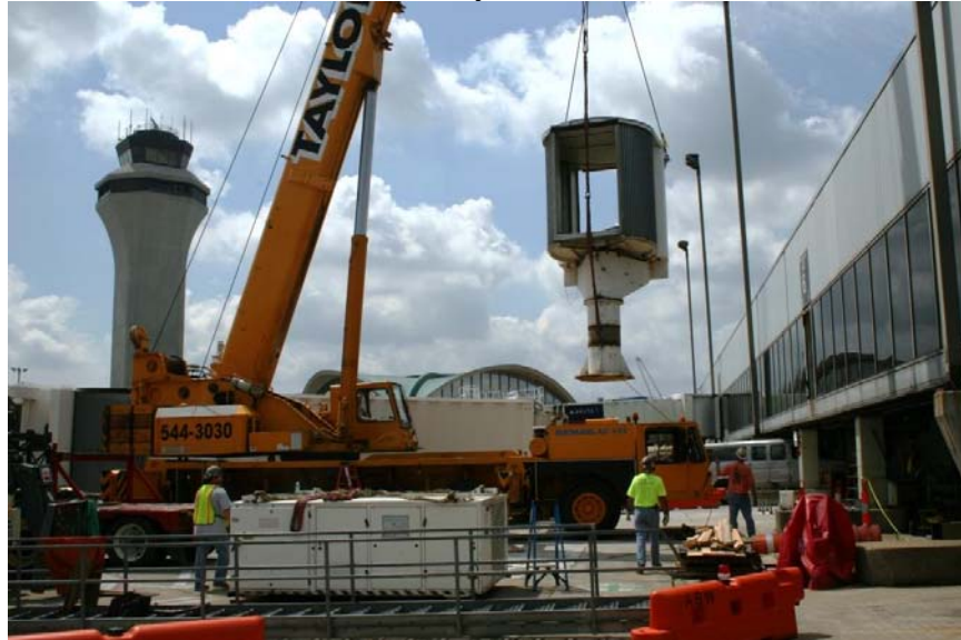
Iron workers guide a loading bridge rotunda into a new foundation at gate A6.
