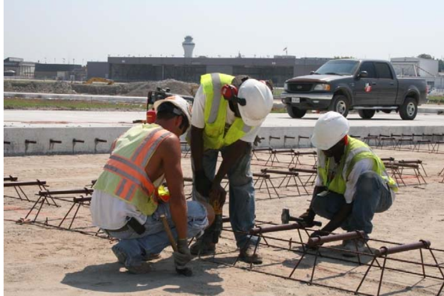
A Millstone Bangert crew works through the heat on the reconstruction of Taxiway Sierra.
