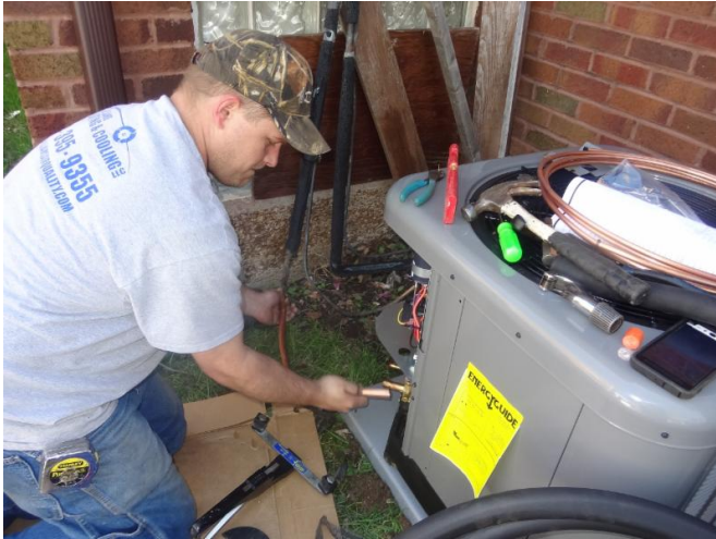
Matt Northway with Williams Heating and Cooling installs two ton air conditioners.
